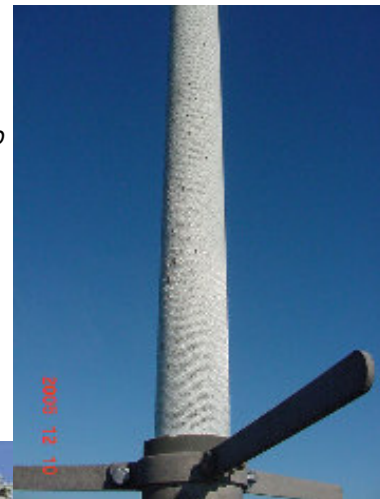
Right: Base of the 70 cm repeater antenna. Photo by Sherrick KA6NZB , taken while atop the antenna pole
